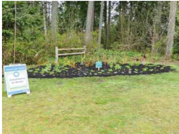
33 - Installation of native plant garden for bat and pollinator species at Westhill Park.
